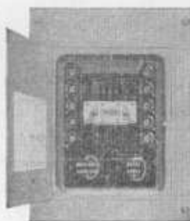
100 Ampere Main And Range Pull Switch
